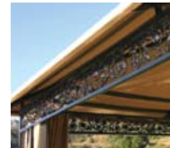
Perimeter wrought iron rigid valance.
