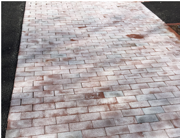
Picture: Efflorescence Caused By Rock Salt De-Icing Salt
